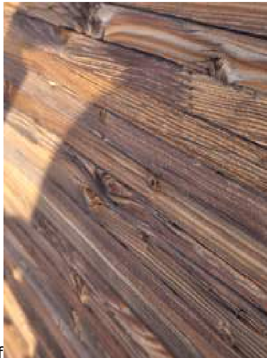
Figure 2B: View of typical weathering of glulam beams
