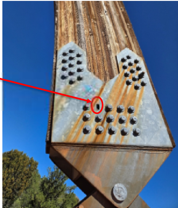
Figure 2C: View of missing bolt in base connection
