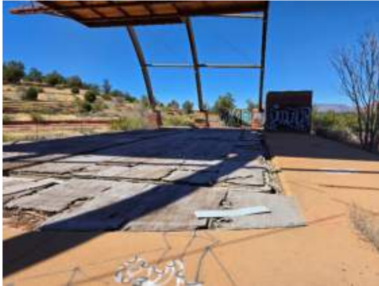
Figure 2G: View of deterioration of stage subfloor
