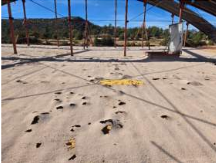
Figure 2I: View of deterioration of membrane roof
