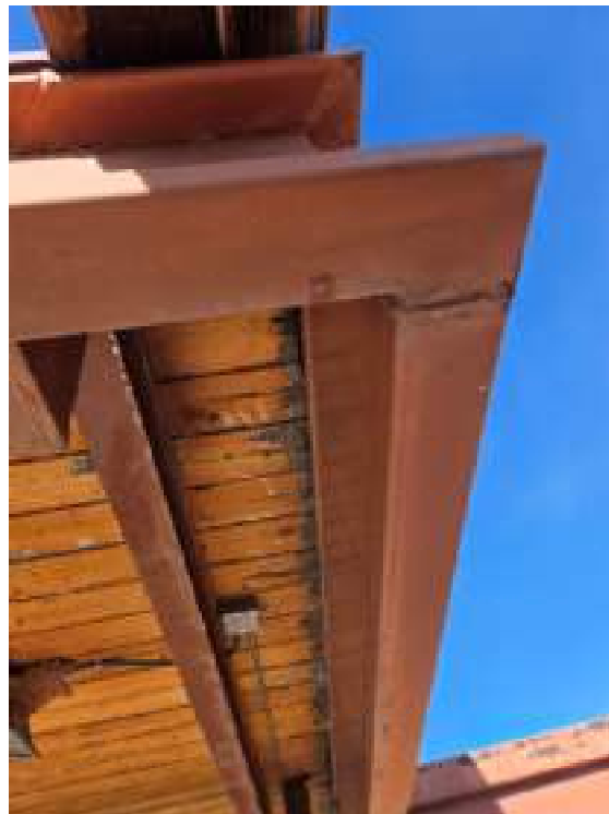
Figure 2J: View of rotting of wood decking
