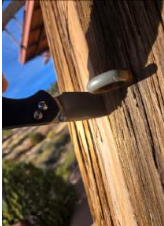
Figure 2A: View of the dry rot at east end of north beam (knife is embedded approximately 2")
